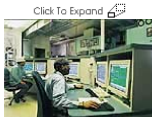
Operator consoles in the control room, old pneumatic control
